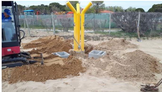
Figure 6.3.5 Showers installed in marina Bibione
