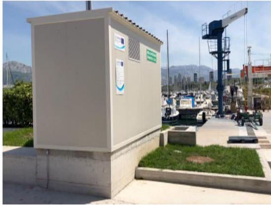
Figure 6.3.3 Physical-chemical purifier of wastewater installed in marina Špinut
