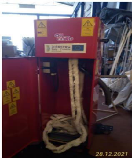
Figure 6.3.6 Mechanical oil separator in marina Porto Baseleghe
