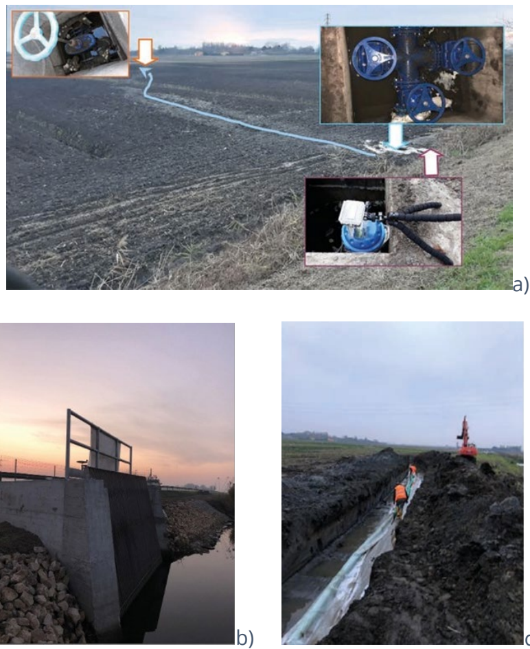
Fig. 13 – Photos of a) the MoST site with the trace of the buried drainpipe and detail of the manholes with valves and flowmeter; b) the realized intake structure; and c) the pipe drain during the installation works.
