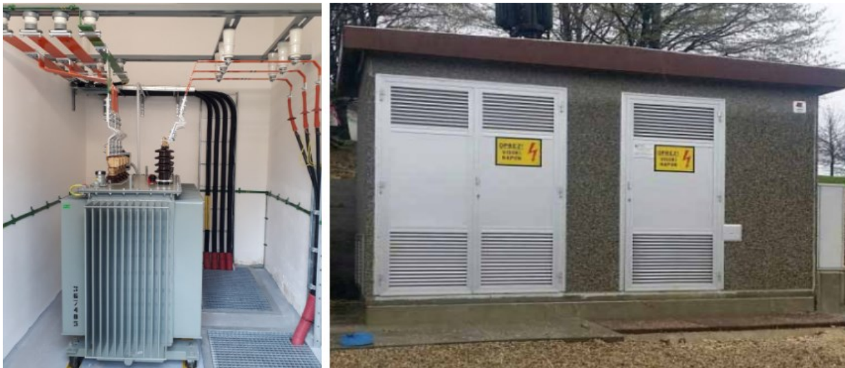
Figure 3. Standard 1000 kVA MV/LV transformer and typical KTS type TS
