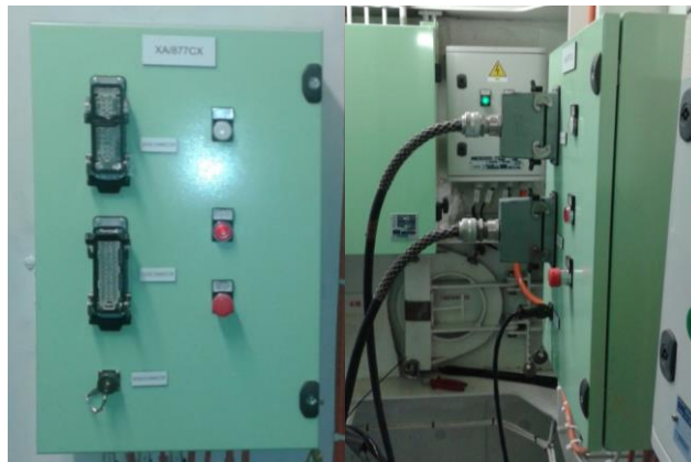
Fig. 5. Shore Connection control cabinet [14].
