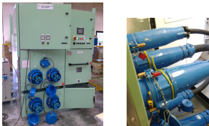
Fig. 3. Typical switchboard for Shore Connection purpose [14].
