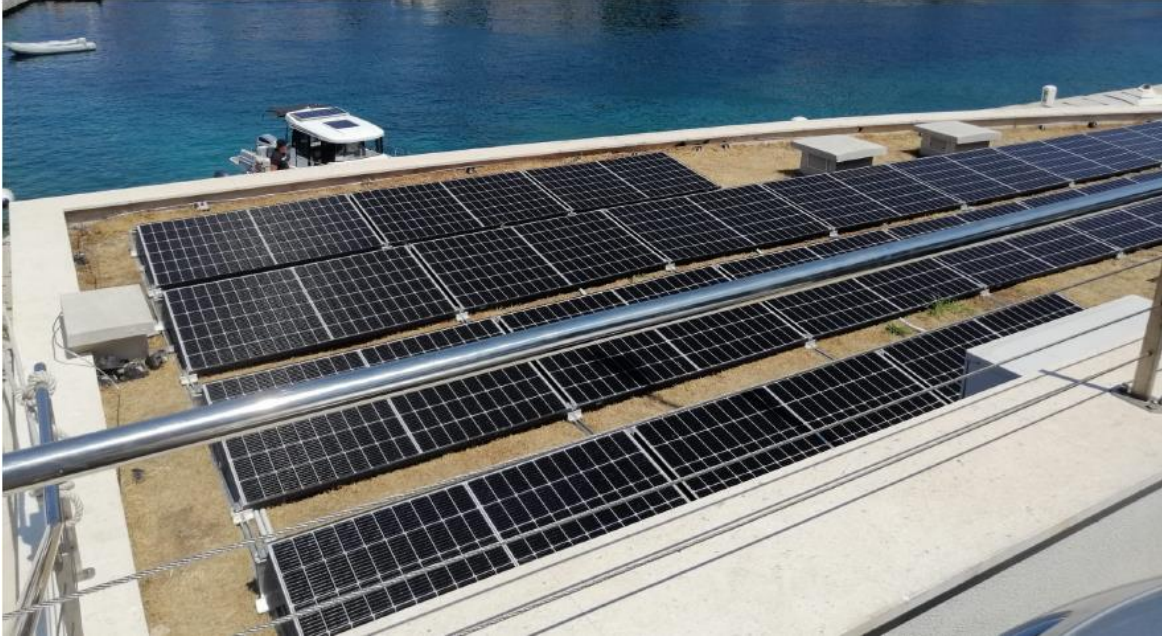
Figure 3 – Micro-grid system installed by PP10 Dvorac.
