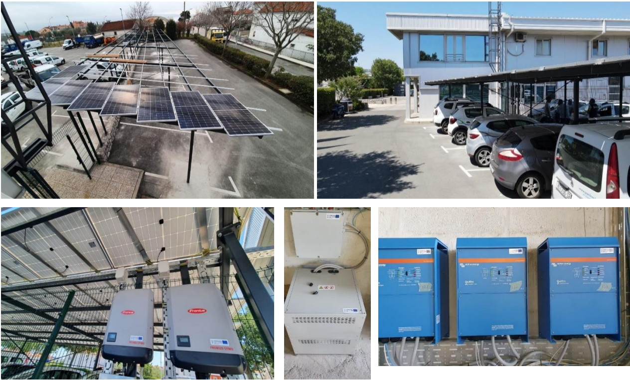
Figure 2 - Micro-grid installed by PP12 Ponikve.
