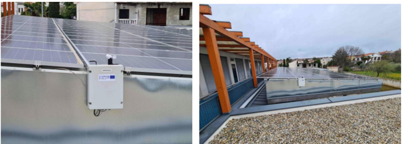
Figure 1 – Micro-grid installed by PP06 in the Municipality of Malinska-Dubasnica.
