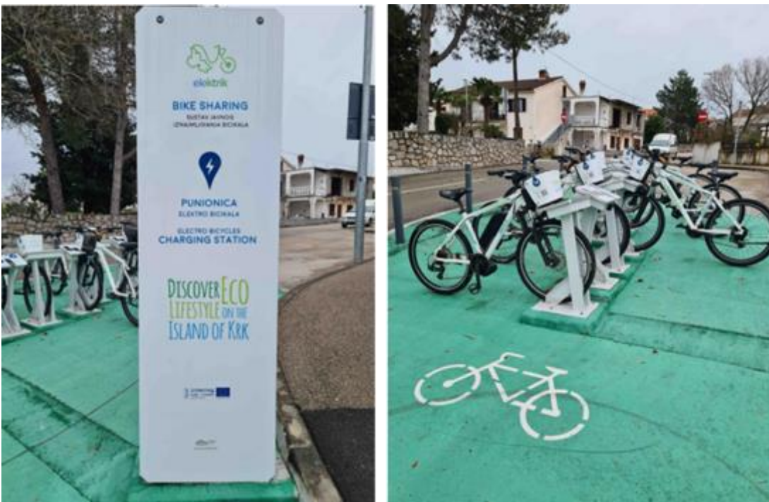
Figure 5 – Bike racks installed in the Municipality of Malinka-Dubasnica on Krk Island by PP06 Malinska.
