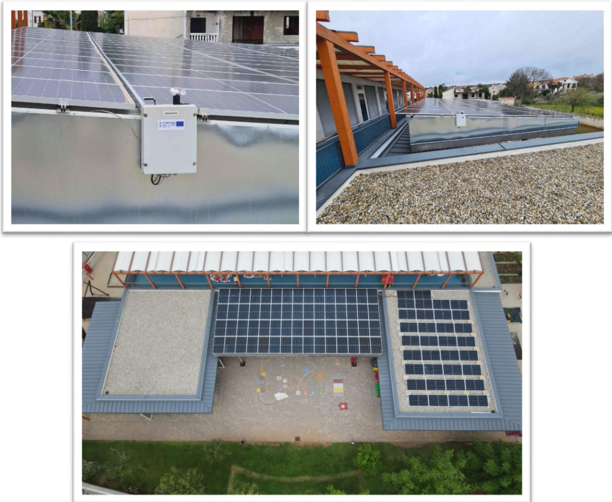
Figure 4: Micro-grid system for e-vehicles and e-boats in Malinska installed by PP06 Municipality of Malinska
