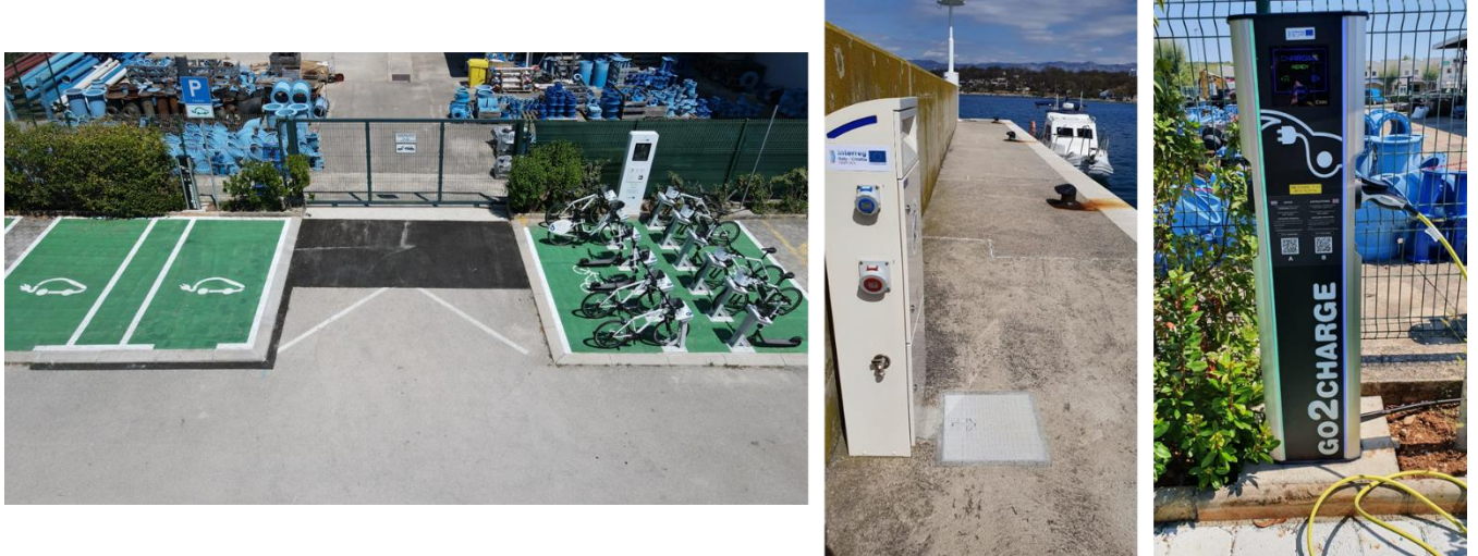
Figure 3: 3 e-charging stations for e-cars and/or e-boats installed by PP12 Ponikve Eco Island of Krk
