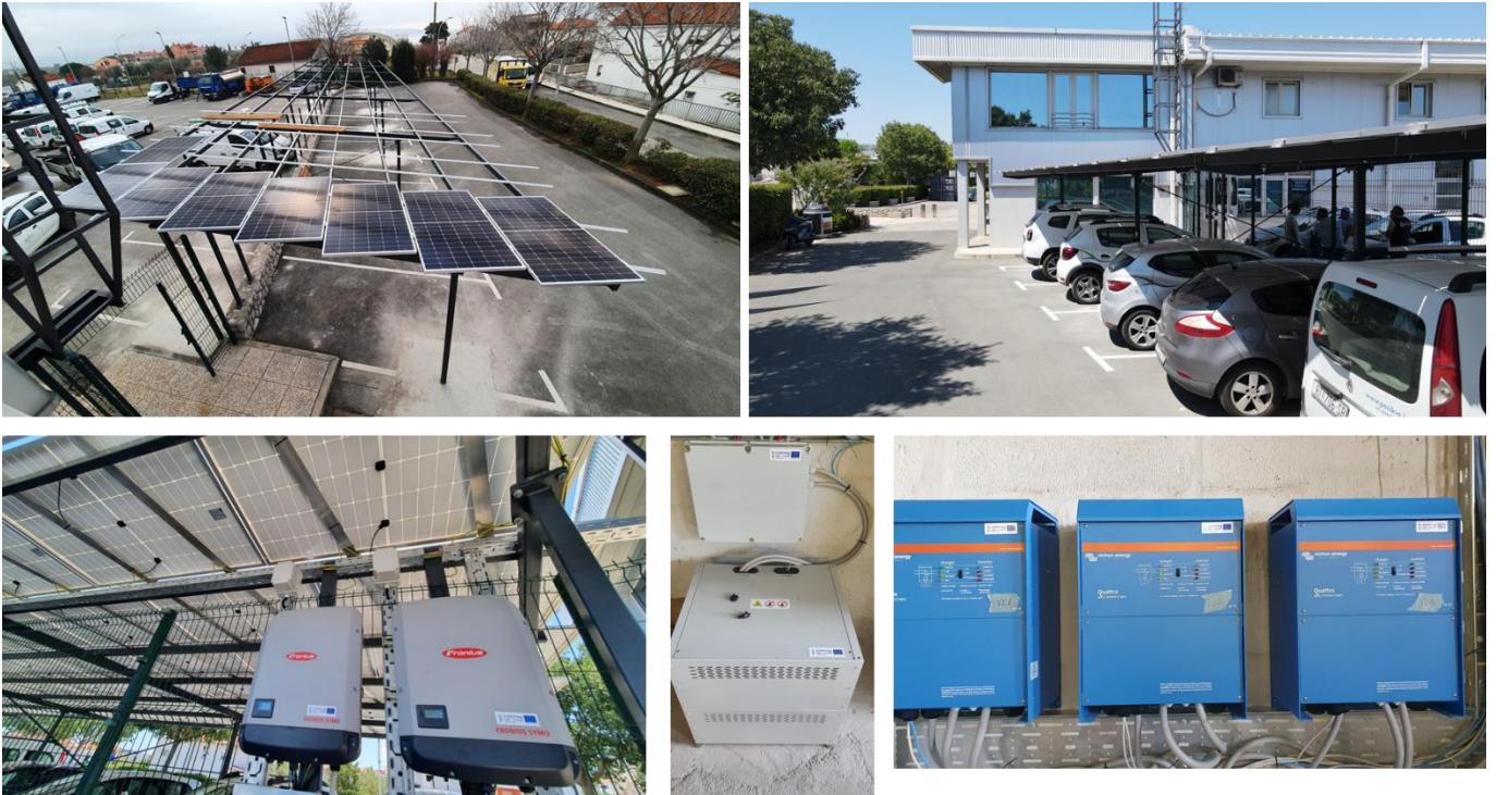
Figure 4: micro-grid system installed by PP12 Ponikve Eco Island of Krk
