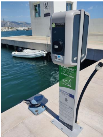
Figura 8 e-charging station, manfredonia
