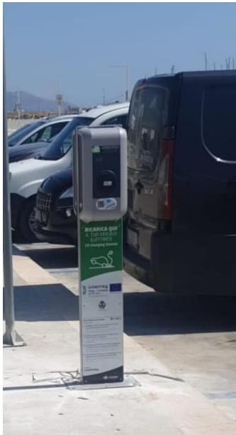
Figura 9 e-charging station, Manfredonia
