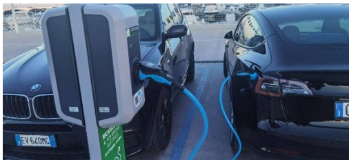
Figura 7 e-charging station Manfredonia
