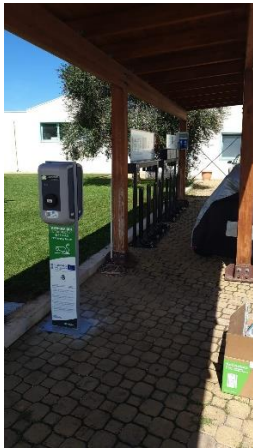
Figura 6 E-charging station, rodi garganico
