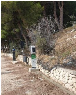
Figura 5 E-charging station, mattinata
