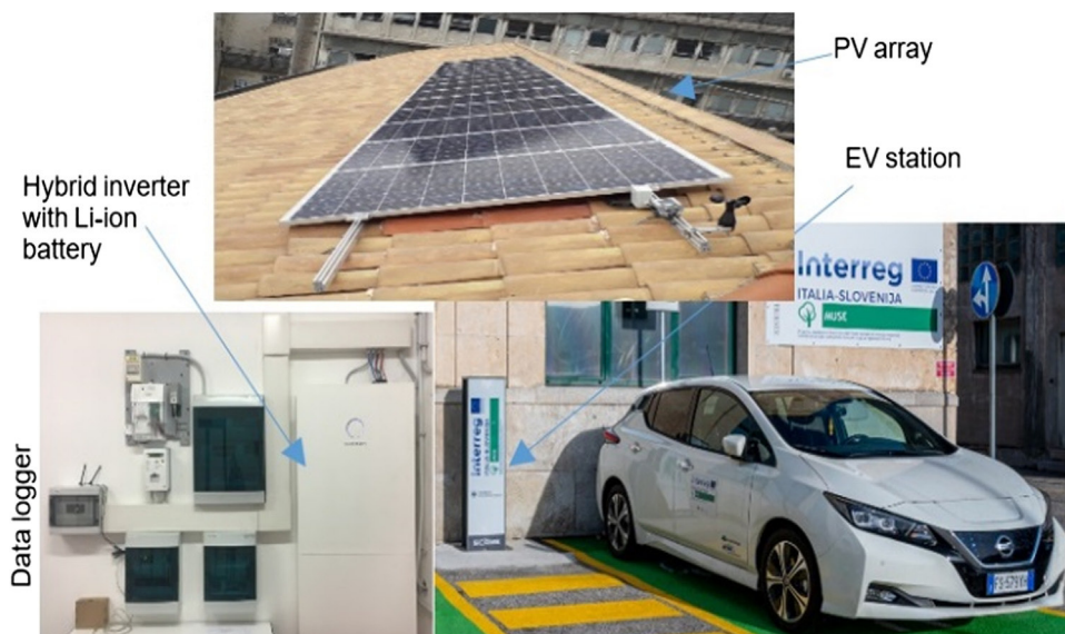
Fig. 1. Key components of the MG investigated in this work, including the 4 kW PV array and the data logger.
