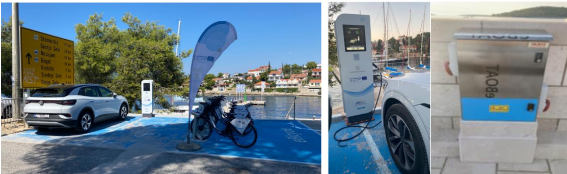
Figure 1 – E-charging station for e-vehicles and e-boats installed by PP10 Dvorac at Martinis Marchi marina.
