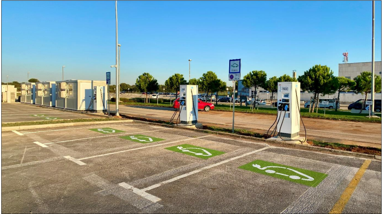
Figure 3. Terra 54 multi-standard DC charging station
