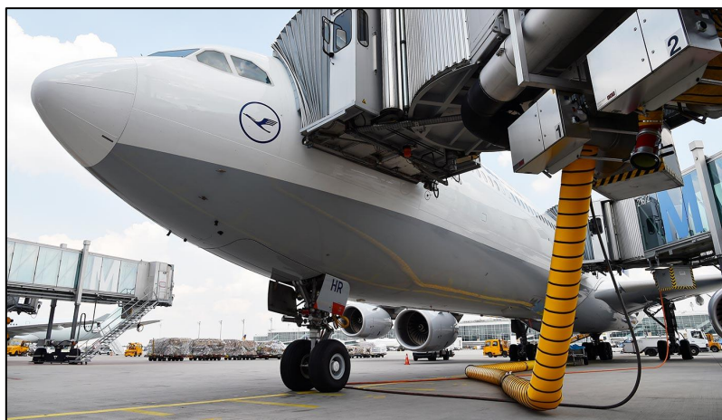
Figure 4. Pre-conditioned air system at Munich Airport 7 .
