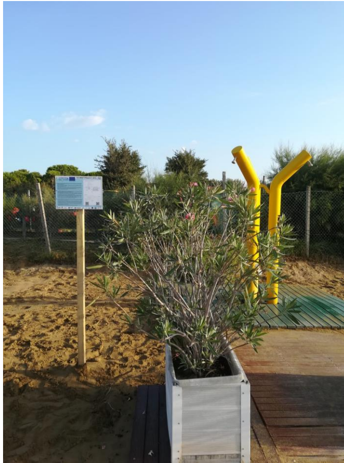
Figure 5. Bibione Mare, eco-showers for water recycling
