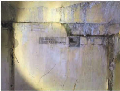
Original writing on the wall, indicating the function of the room and showing the ventilation tube
