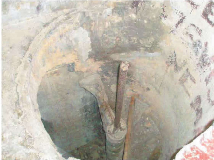
2.7. Remains of concrete spiral stairs.
