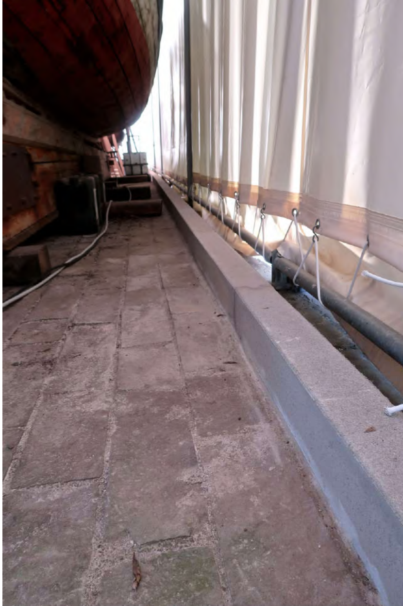
The concrete curb to prevent rainwater from flowing the floor.
