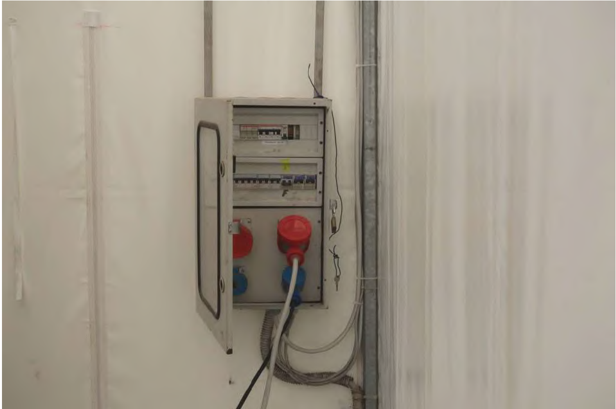
The new electric panel and the related new electric system.
