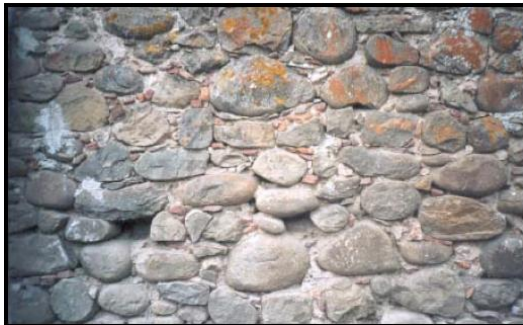
DESCRIPTION: Wall composed of rounded stone with polished surface and without layers with inserts of bricks.
