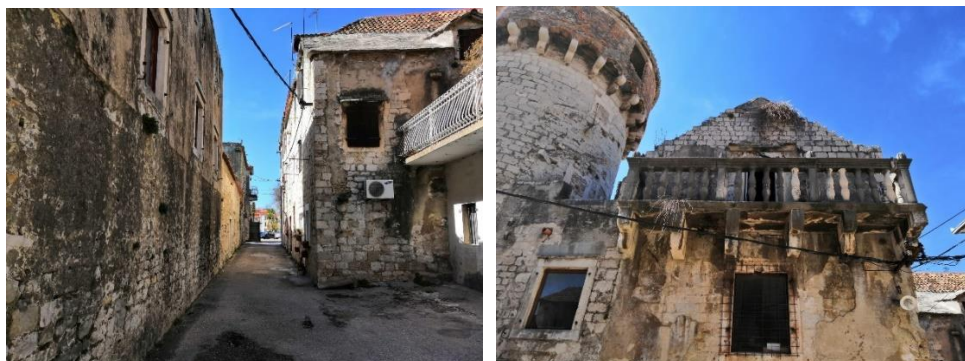
Fig. 10. Damaged buildings in the historical centre
