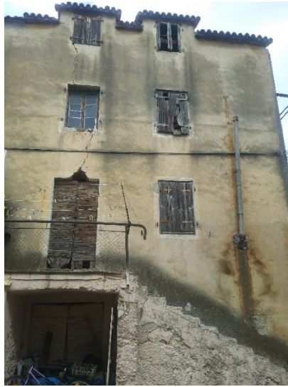
Fig. 13. Building with significant cracks
