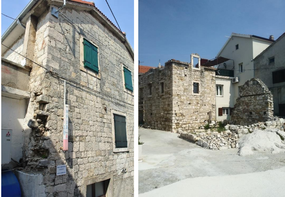
Fig. 11. Damaged walls and destroyed roofs of the buildings
