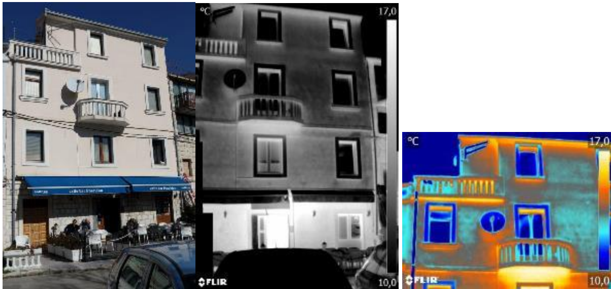
Fig. 22. Residential building Drage Britvića 13: Stone masonry walls with RC floors, balcony and roof slabs is characteristics of reconstructed old stone masonry building.
