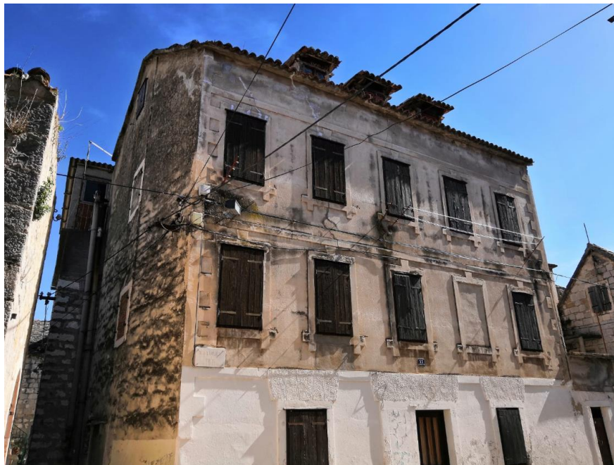
Fig. 12. Uninhabited building in the centre with significant cracks
