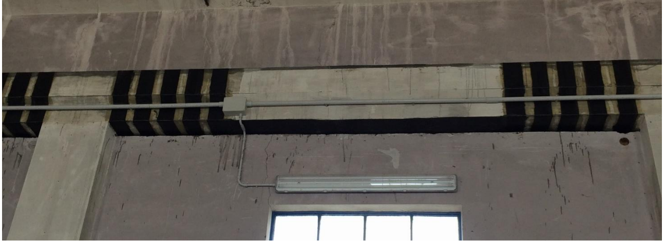
Figure 31. Damage state of the r.c. beams.
