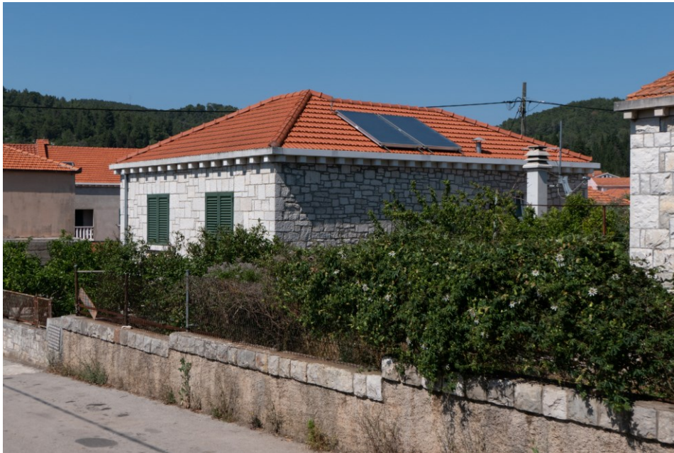
Study visit - solar collector on house rooftop in Vela Luka
