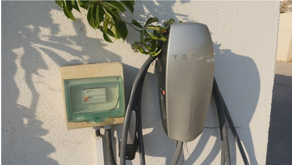
Study visit – Electric charging station in Lumbarda
