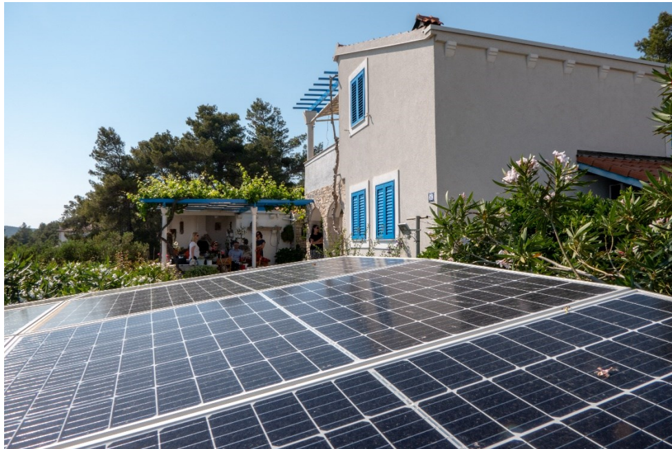
Study visit - solar photovoltaic panel serving as garage rooftop in Vela Luka
