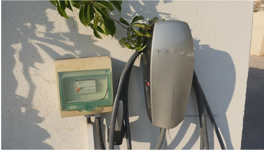
Study visit – Electric charging station in Lumbarda
