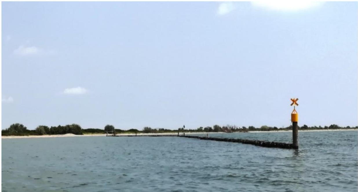
Figure 17. Diversion barrier at the seaside of the outer sand bar of Sacca di Goro.
