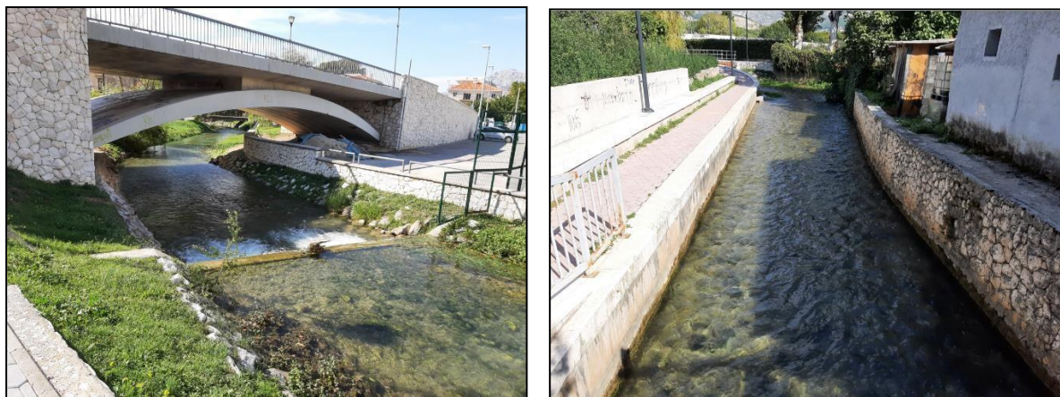
Figure 9. The Jadro river banks and beds in lower course of the river
