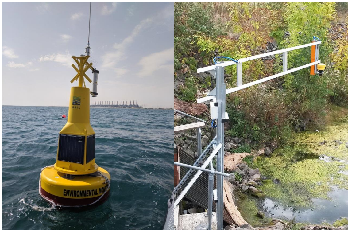
Figure I-6. Examples of petroleum or oil detection sensor installation
