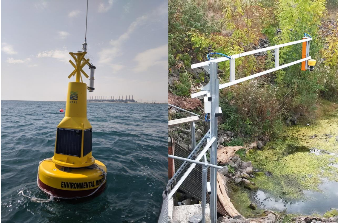
Figure 3. Examples of oil detection sensor installation
