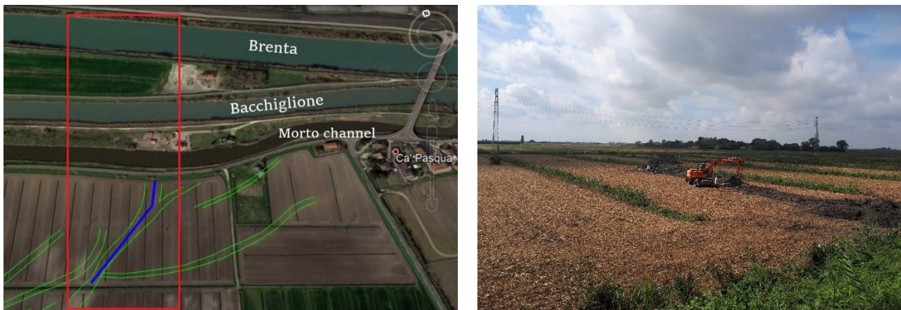
Figure 2.2 Trace of the recharge drain (line in blue) along the main paleochannel (in green) in the study area delimited in red (to the left) and the drain installation during the field operations (to the right).
