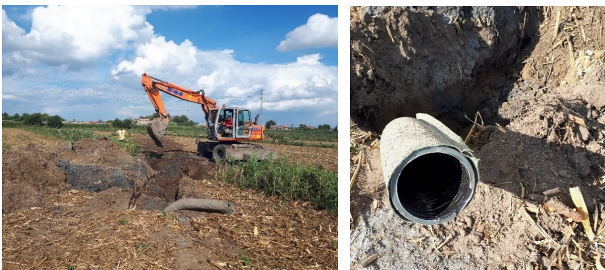
Figure 2.3 Detail of the drain location along the paleochannel (to the left) and of the drain (to the right).
