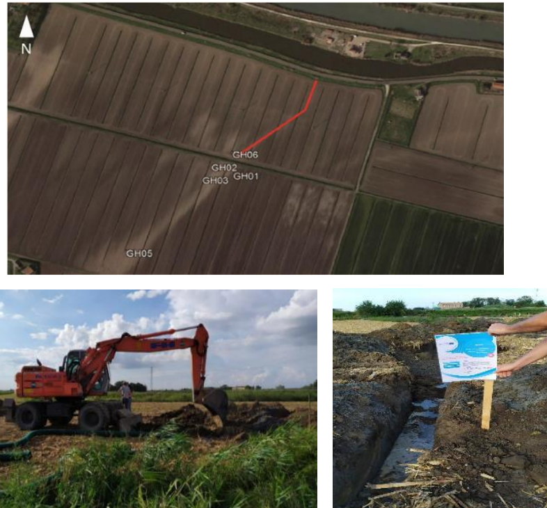
Fig. 4 – a) location of the surficial sedimentary cores and position of the trench used for the installation of the sub-irrigation pipe (red line); b) and c) photos of the digger at work and the trench.
