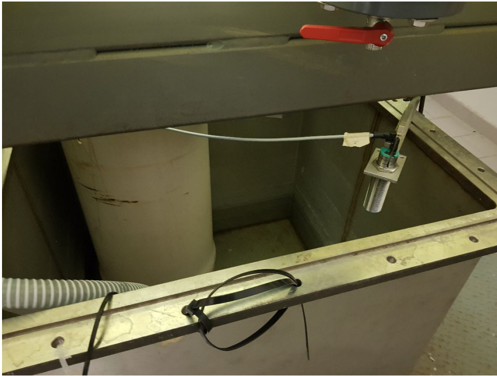
Figure 12 - Sensor system of the downstream metering tank: downstream view
