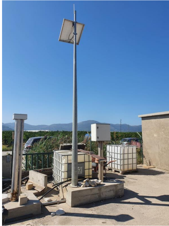
Figure 17 Monitoring location GW_MON_D3
