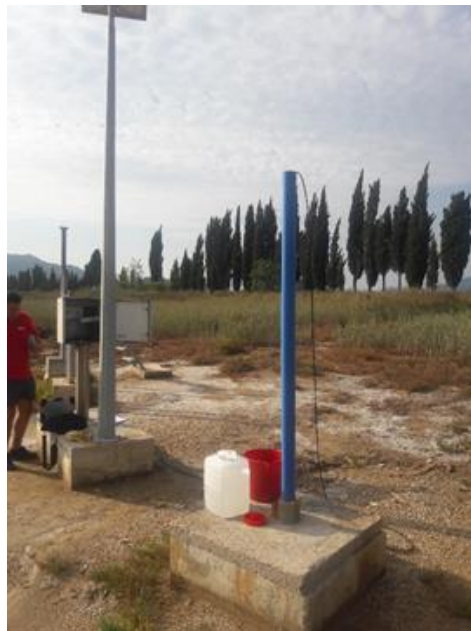
Figure 4 Existing piezometers tested for functionality at Neretva site
