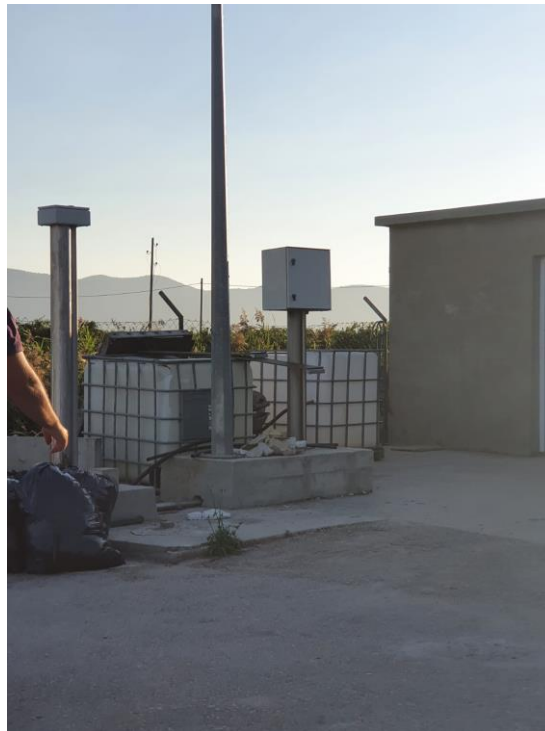
Figure 16 Monitoring location GW_MON_D3
