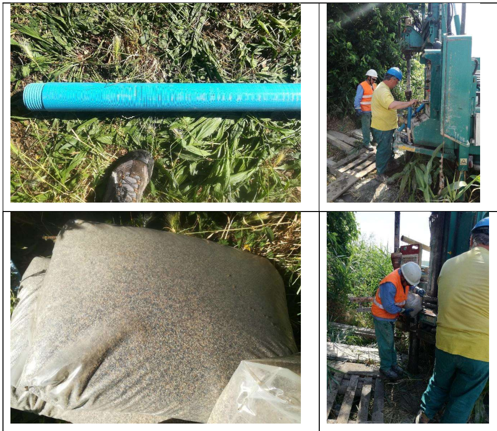
Fig. 9 – Screened pipe and gravel used to fill the pipe soil interspace in new MoST piezometers.
