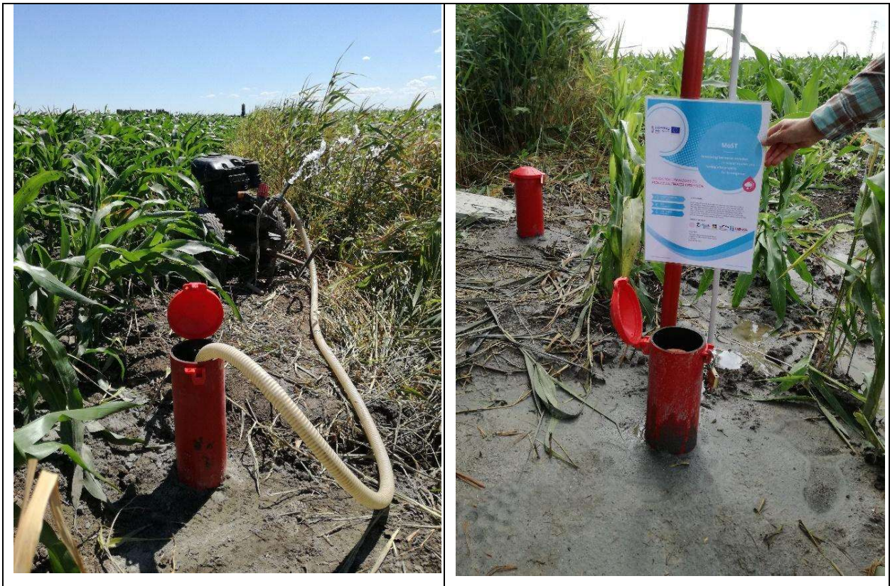
Fig. 10 – a) cleaning of a new piezometer (MoST2), b) final setup of MoST1a and MoST1b piezometers.
