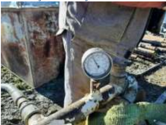
Figure 8.3 Injection flow and pressure meter
