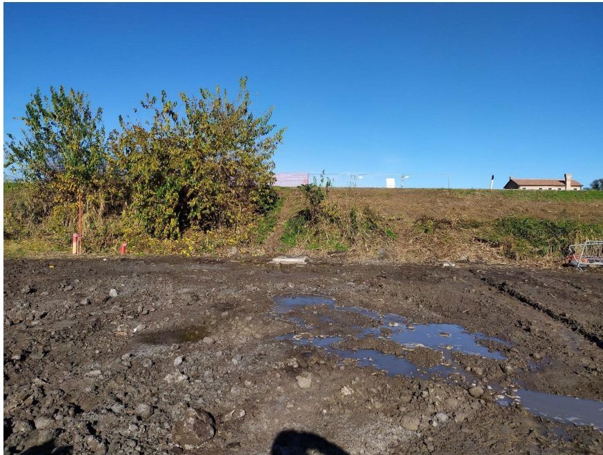
Fig. 24 - The northernmost part of the test area flooded during the operation of the pipe, due to a breakage of the sub-irrigation-pipe.
