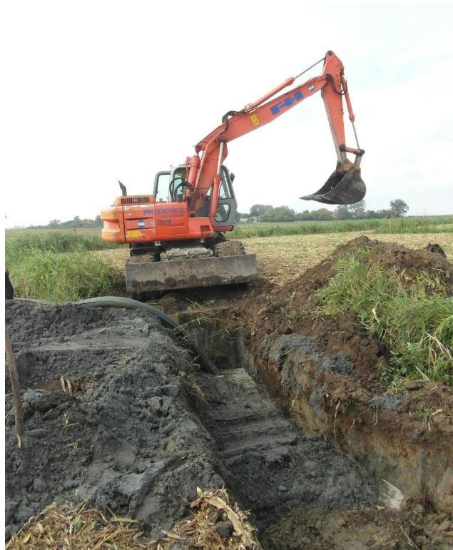
Fig. 14 - Excavator working for the excavation of the trench and positioning of the pipe.
