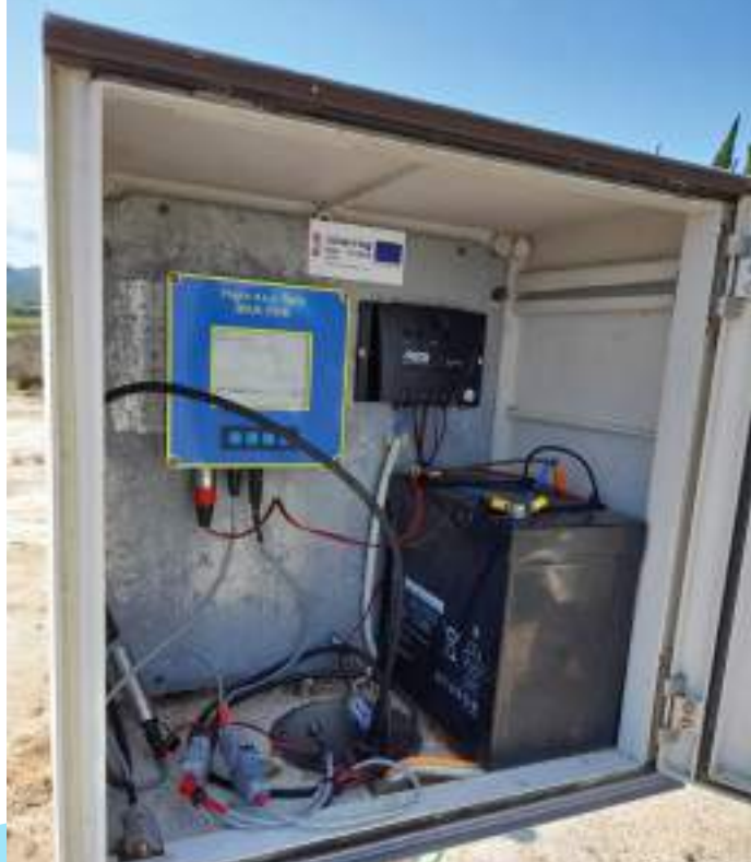
FIGURE 10. INTERIOR OF THE MONITORING BOX AT THE PIEZOMETER
