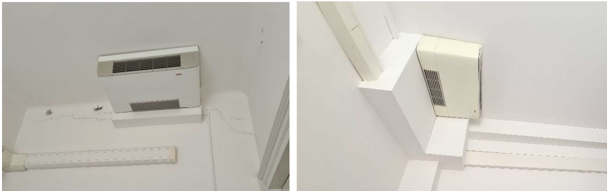
Figure 7. Existing fan coils
