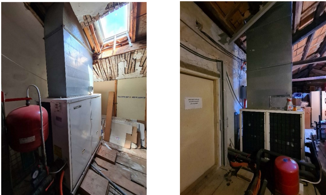
Figure 6. Heat pumps in the attic
