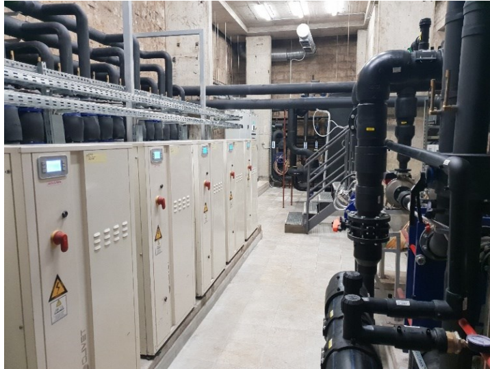
Figure 55 - Heat pump installation in Rector's Palace
