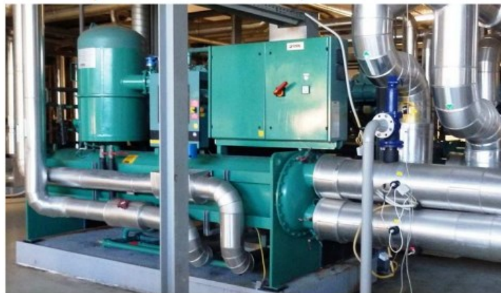
Figure 51 - Heat pump system for the Hotel Punta Skala, Zadar
