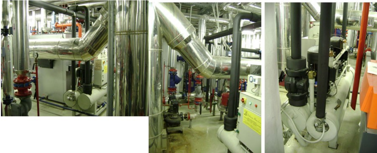
Figure 50 - Heat pump system for the Hotel La Meridien Lav, Podstrana
