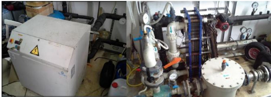
Figure 34 - A heat exchanger and pipeline system
