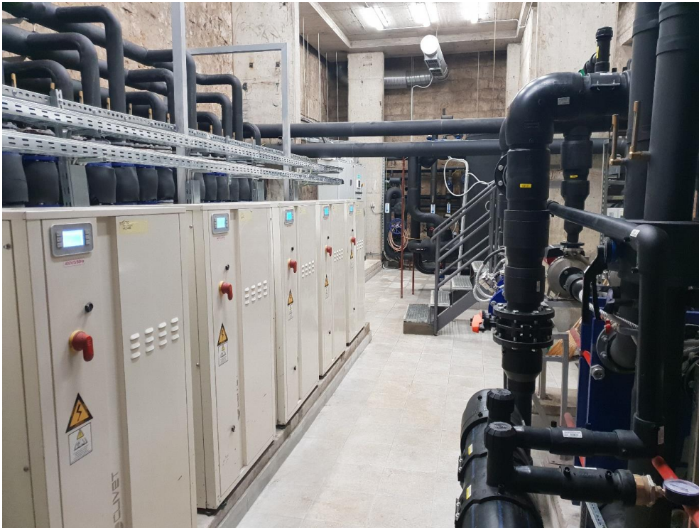
Figure 37 - Heat pump installation
