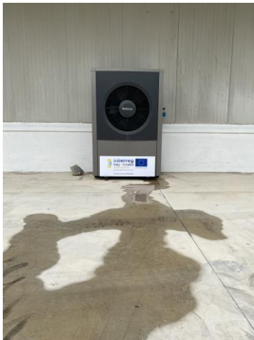
Picture 3 - heat pump engine
