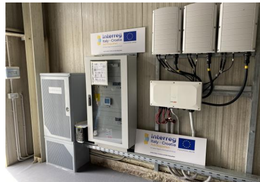
Picture 2 - heat pump equipment
