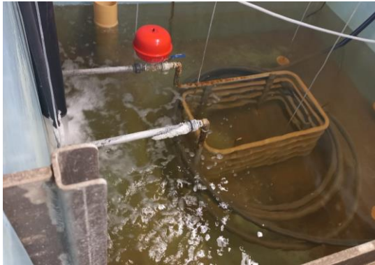
Picture 1 - Prototype water heater installed in Ittica Caldoli
