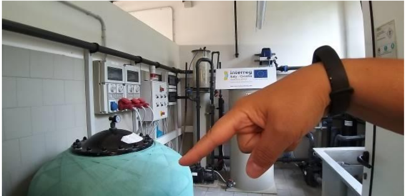
Mechanical sand filter connected to the RAS system used to remove solid waste particle form the water.
