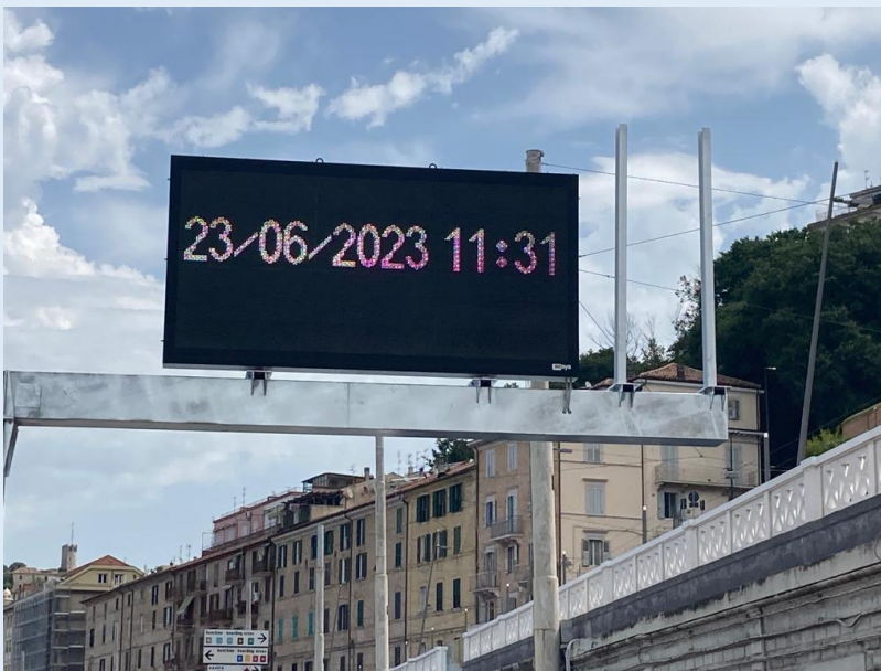
Gate "Varco Da Chio" new MIMOSA LED panels
