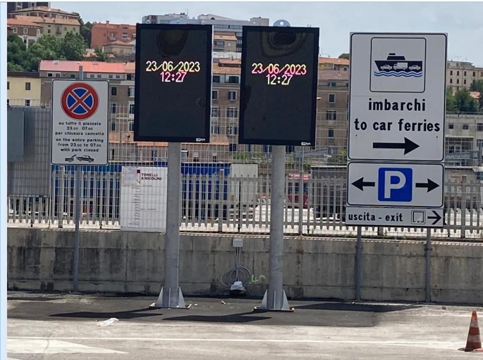
Ticketing terminal new MIMOSA LED panels
