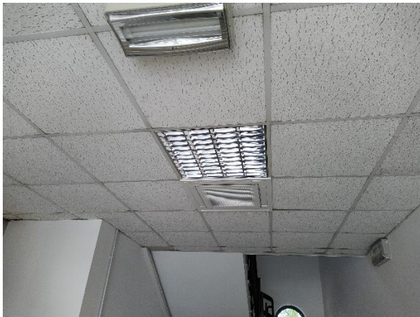
08 Internal air conditioning units
