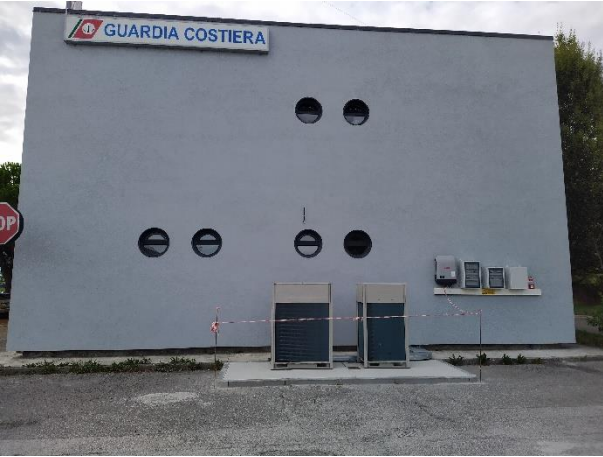
07 Inverter and external air conditioning units
