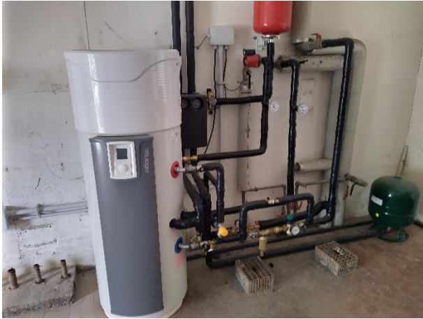
10 Thermal Central Boiler
