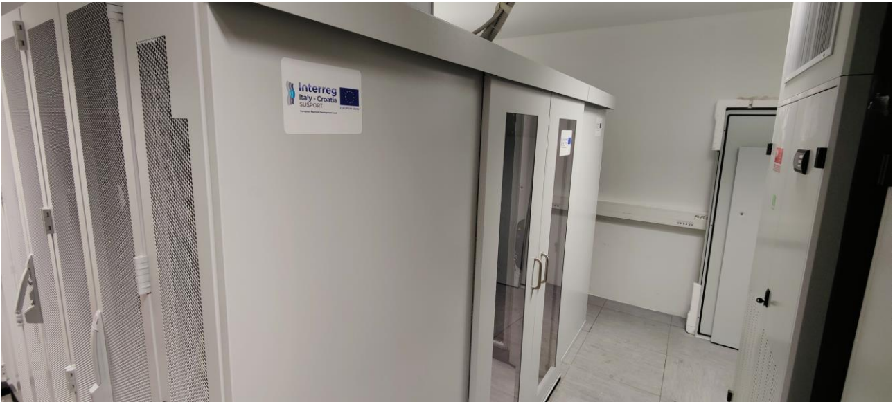
Figure 7 Air condition system
