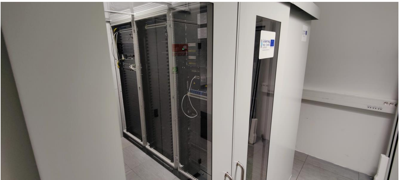
Figure 8 Air condition system
