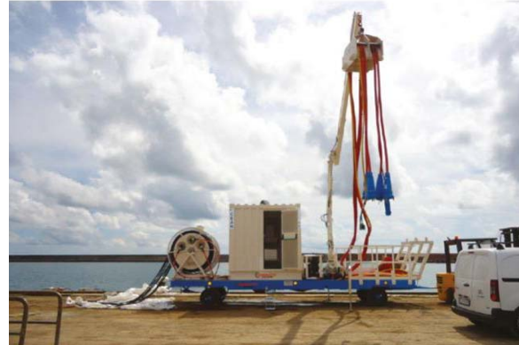
Fig. 4. Mobile structure for ships' cold ironing in the port of Genoa (Source: Port System Authority of the Western Ligurian Sea)
