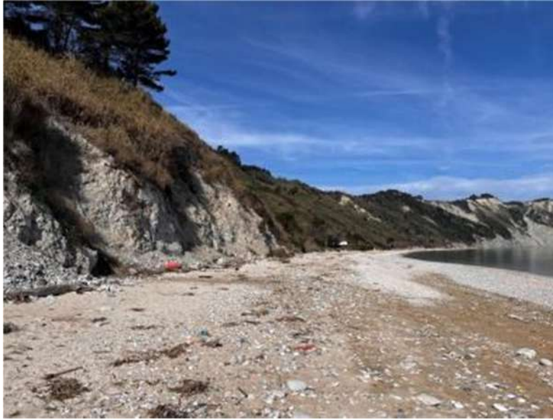
Figure 130. Transept 15_he_404 - Landslides and landslides of the upstream slope
