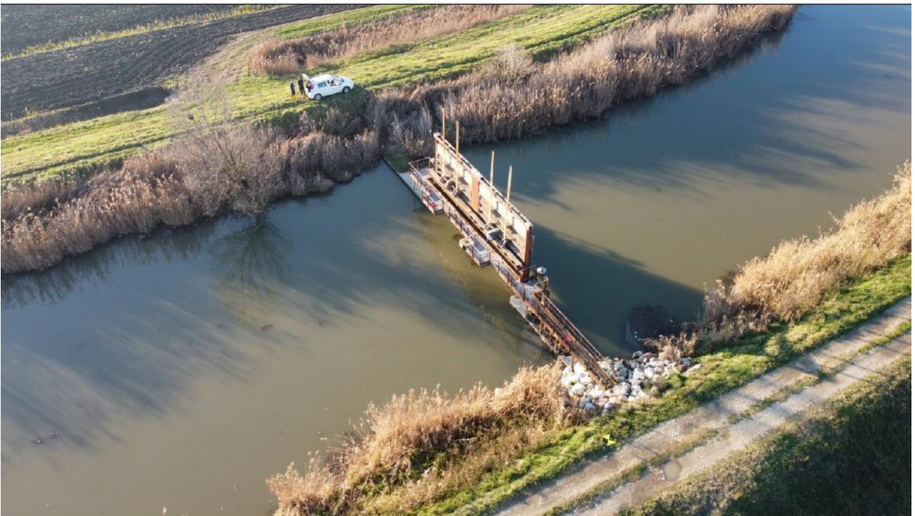
Figure 3: Aerial photo of the portion of Vela Channel interested by the intervention.
