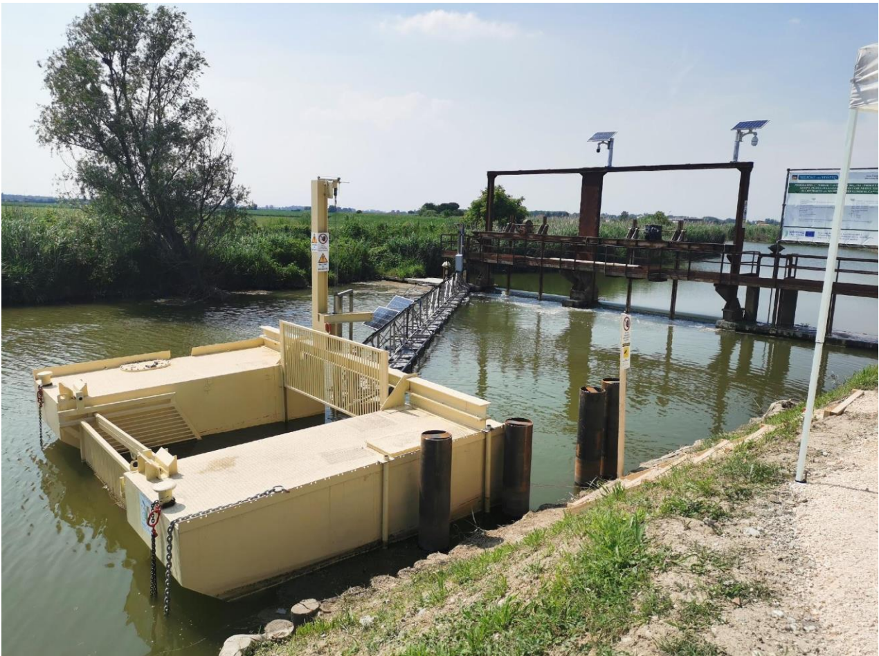
Figure 5: Pilot site with devices in place.
