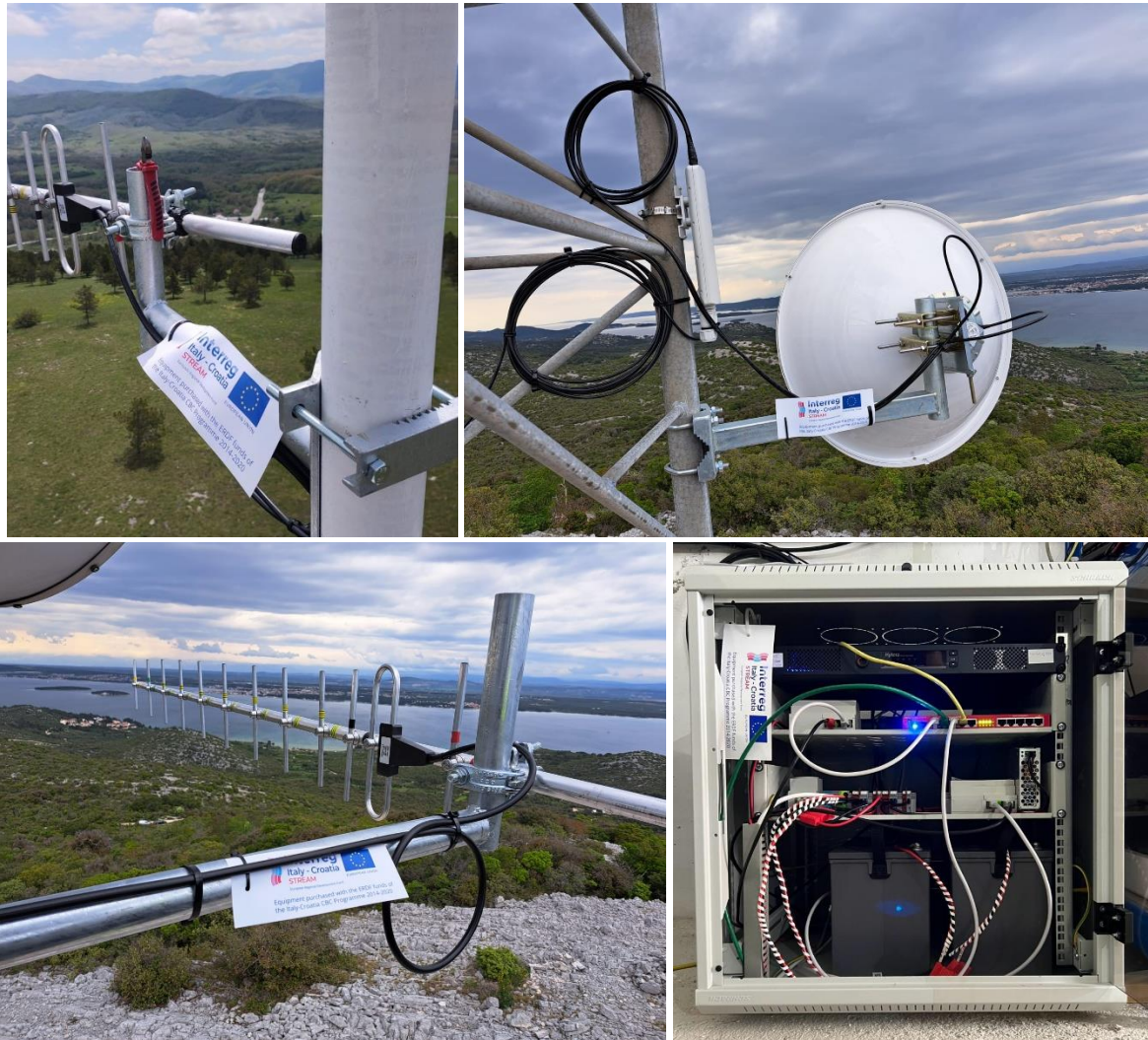
Figure 3. Equipment for the radio-communication system
