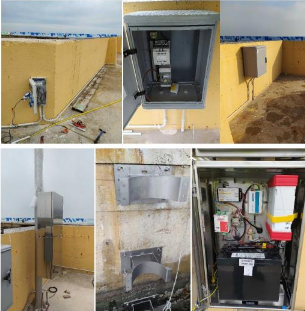
Figure 12. Pictures of the tide gauge installed in Cattolica (RN)
