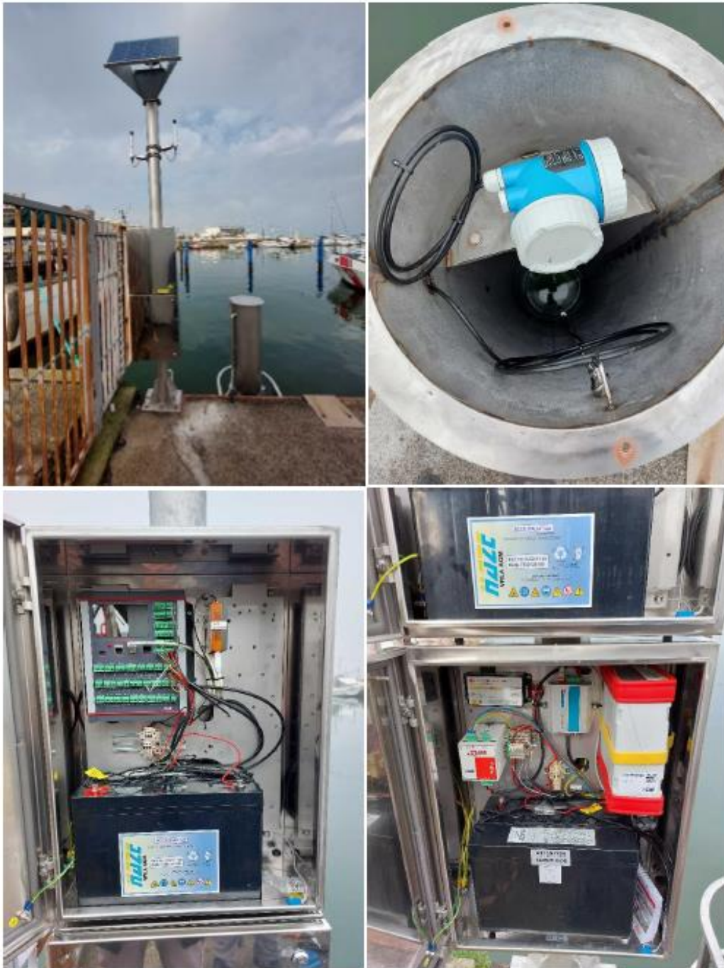
Figure 10. Pictures of the tide gauge installed in Cervia (RA)
