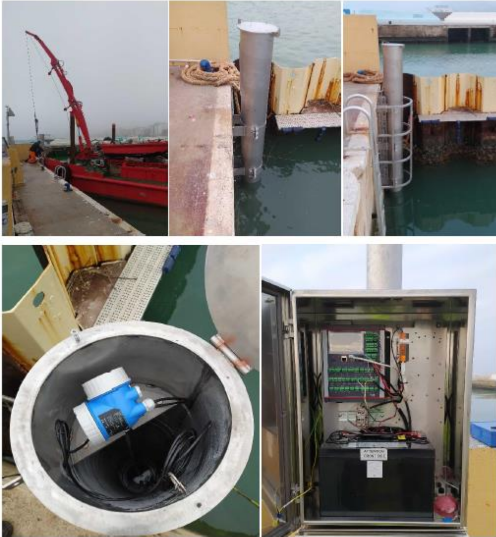
Figure 13. Pictures of the tide gauge installed in Cattolica (RN)
