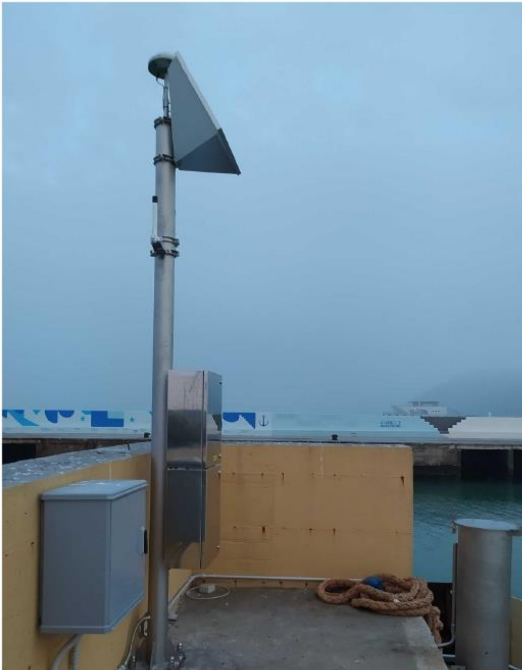
Figure 15. Cattolica tide gauge and GNSS station (RN)
