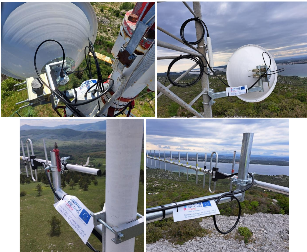
Figure 2. Repeaters installed at 4 locations in Zadar County
