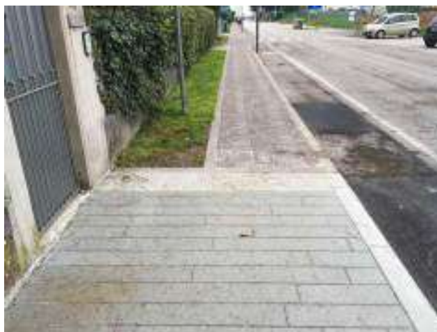
Fig.9 Really dangerous pavement with tactilo-plantar sign.
