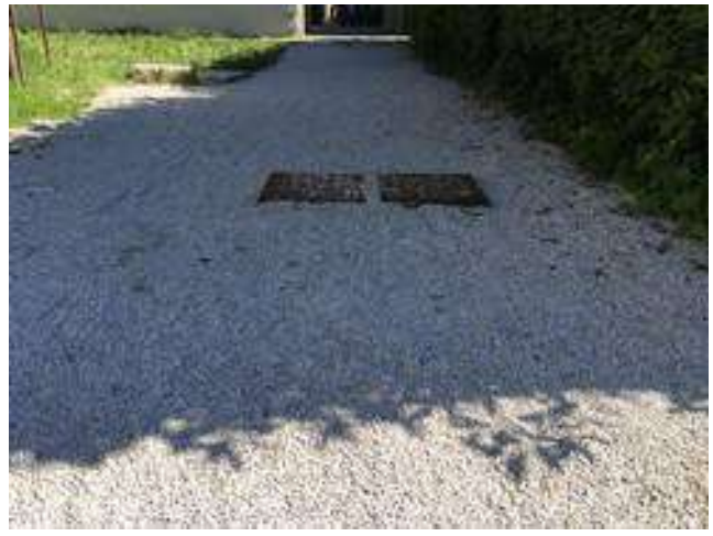
Fig.7 Protruding sewer covers.
