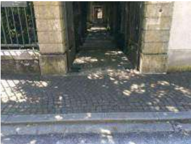
Fig.2 Pavement with a 5 cm step.
