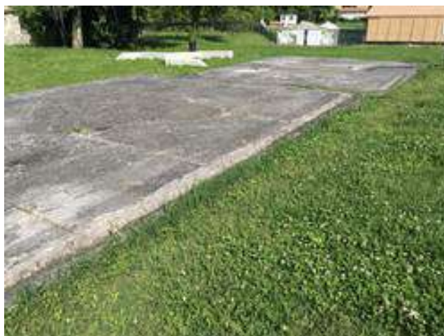
Fig.13 Cement slabs with mosaics deteriorated by atmospheric agents.
