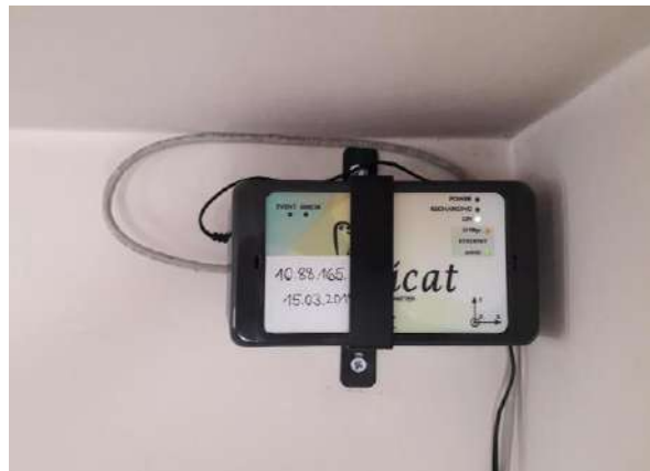
Accelerometer for continuous monitoring
