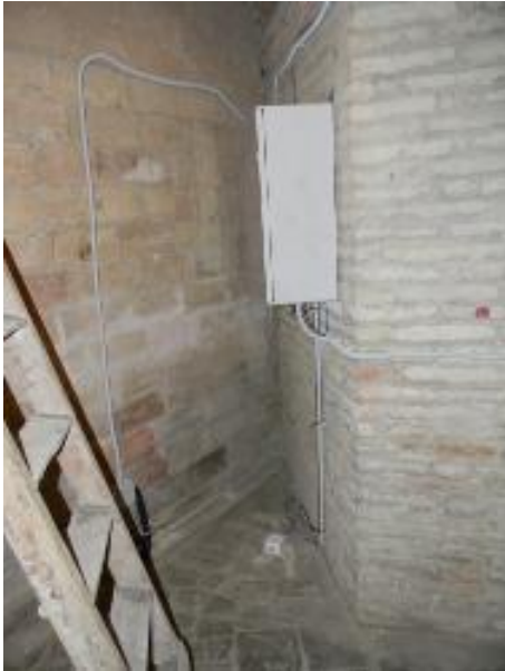
Treia seismic station
